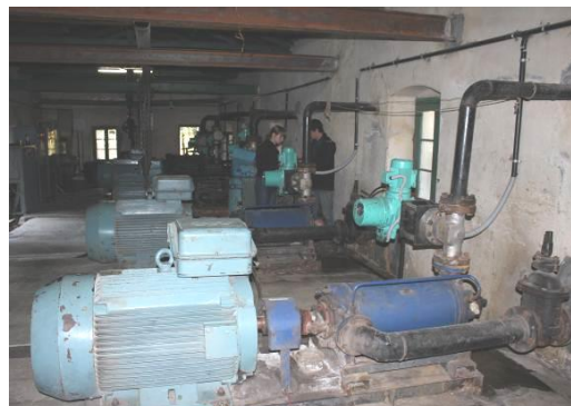
Figure 4. Pump set 6 at Murray Pump Station, with an efficiency of nearly 60%
