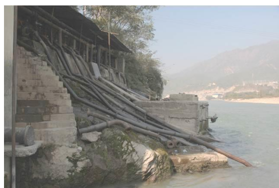
Figure 2. Suction pipes with non-return valves in the River Alaknanda
