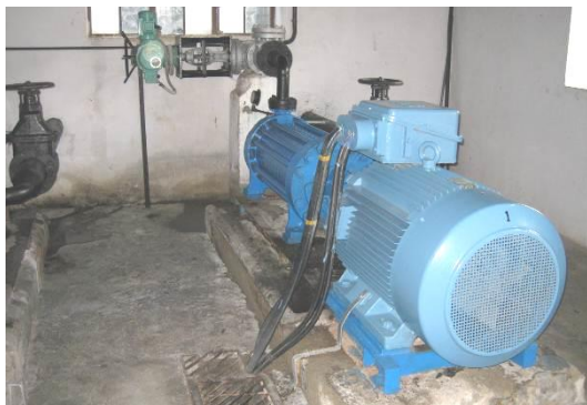
Figure 3. Pump set 1 at Jinsy II Pump Station, wire-to-water efficiency of 47%, Mussoorie
