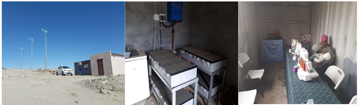
Figure 1. The Benguela Community Wind Energy System comprising the turbines, control room and sewing room
