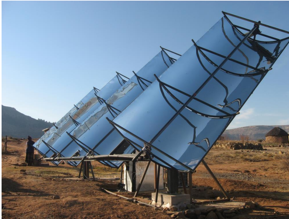
Figure 1. First solar ORC prototype installed by STG in Lesotho
