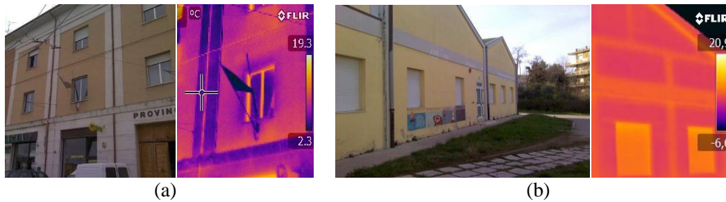
Figure 5. Infrared thermography (IRT) carried out during energy audit activities: Province of Chieti office building at Chieti (a); Nursery School “S. Giuseppe” at Ortona (b)
