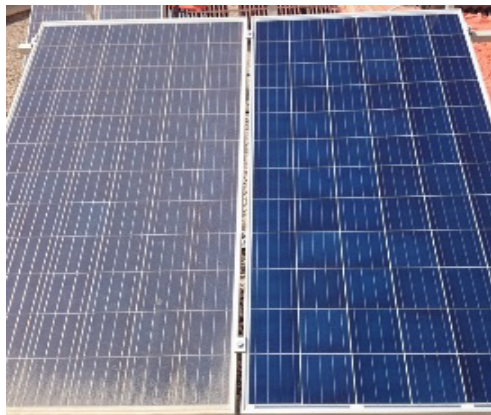
Figure 5. Image of clean and naturally dusted modules.
