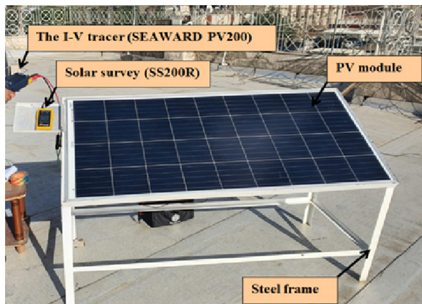
Figure 1. Tested PV module of nominal power 165 W
