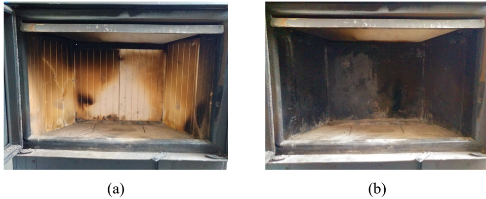
Figure 1. The view of the furnace with complete fire clay layer (a) and partially removed fire clay layer (b)
